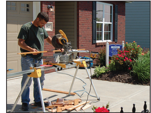
Worker completes trim work at Charleston model homes at 150th and Fort Streets.
